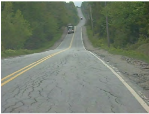
Big Trucks, Rough Roads and Damaged Shoulders
